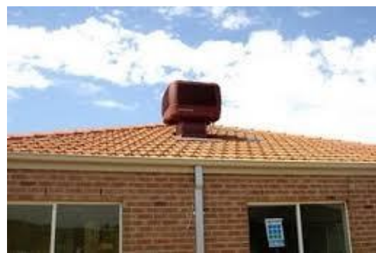
Standard unit in clear view of the street - Not acceptable
